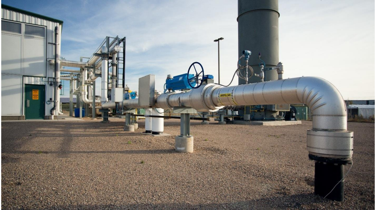
Landfill Gas Collection and Power Generation Facility
