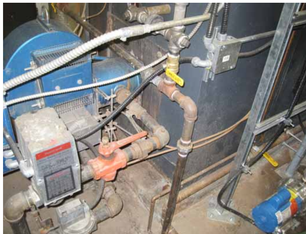
PHOTOGRAPH NO. S11-7721A-10 Natural gas fired boiler system.
