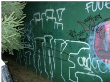
Wall of graffiti vandalism located adjacent to SkatePark.
