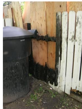
Evidence of previous garbage can fire.
