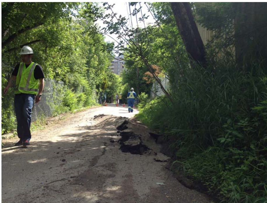
Photo C.6. Bulging Toe of Slide on Cherry Lane (June 21, 2012)
