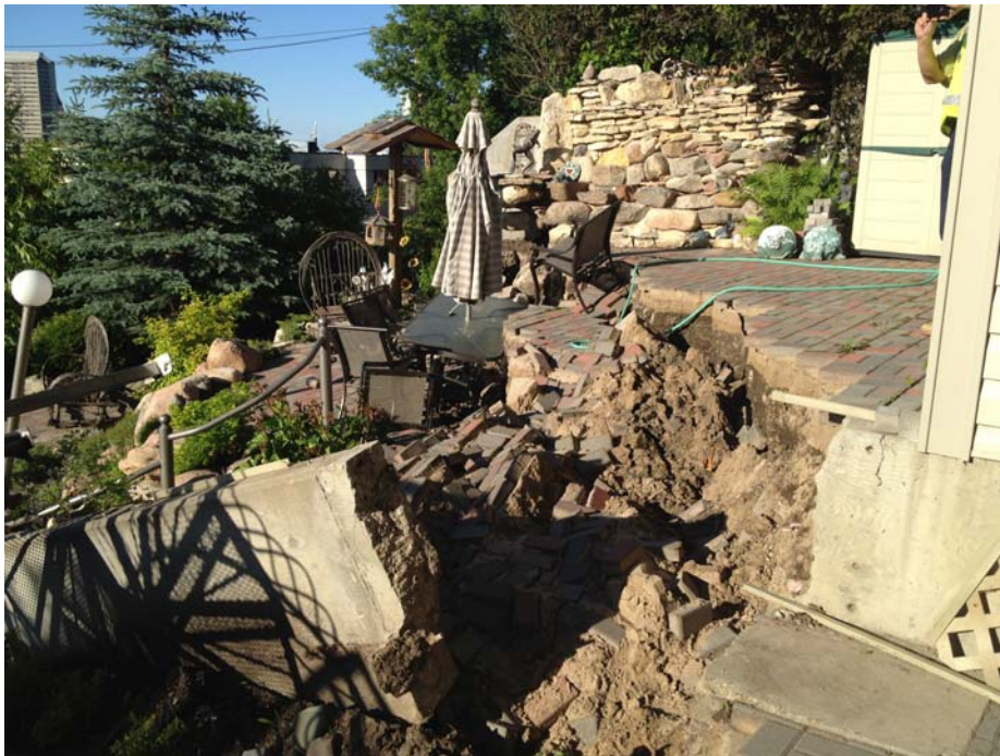
Photo C.5. Headscarp in the Backyard of 233-235 11th St. E. (June 21, 2012)
