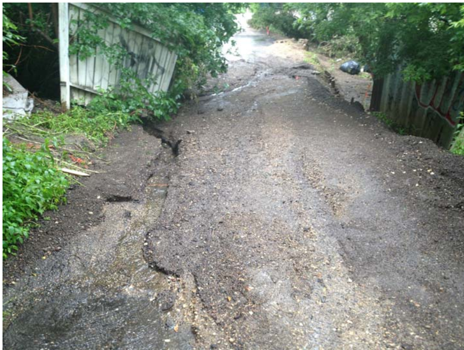
Photo C.22. Looking West at Erosion along Cherry Lane (June 6, 2013)
