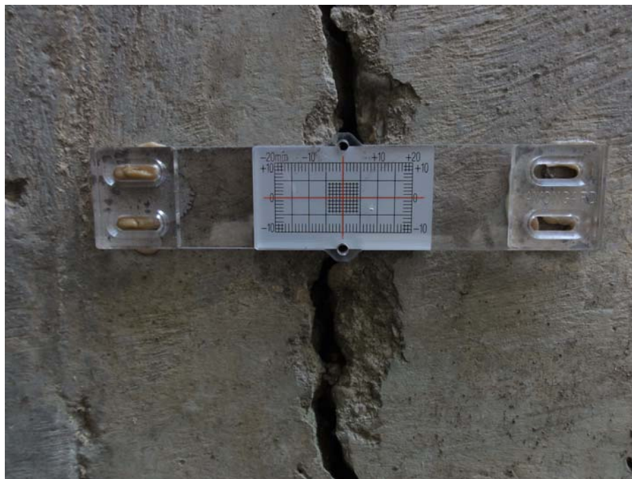
Photo F.2: Crack Meter Located on the Retaining Wall Behind 306 Sask. Cres. E. (CM1) (Sept 18, 2013)
