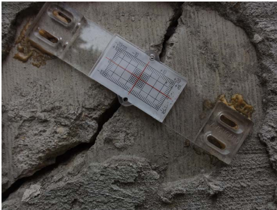
Photo F.4: Crack Meter Located on the East Face of the Retaining Wall Between 230 & 306 Sask. Cres. E. (CM2) (Sept 18, 2013)
