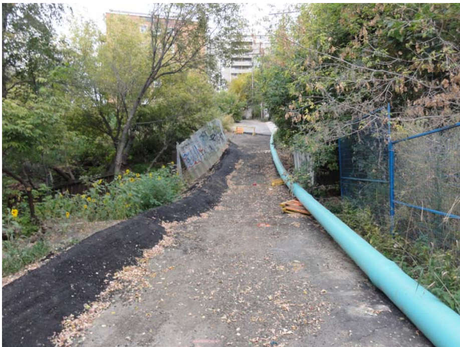
Photo C.29. Looking East at Above Ground Driantage System Installed on Cherry Lane (September 18, 2013)
