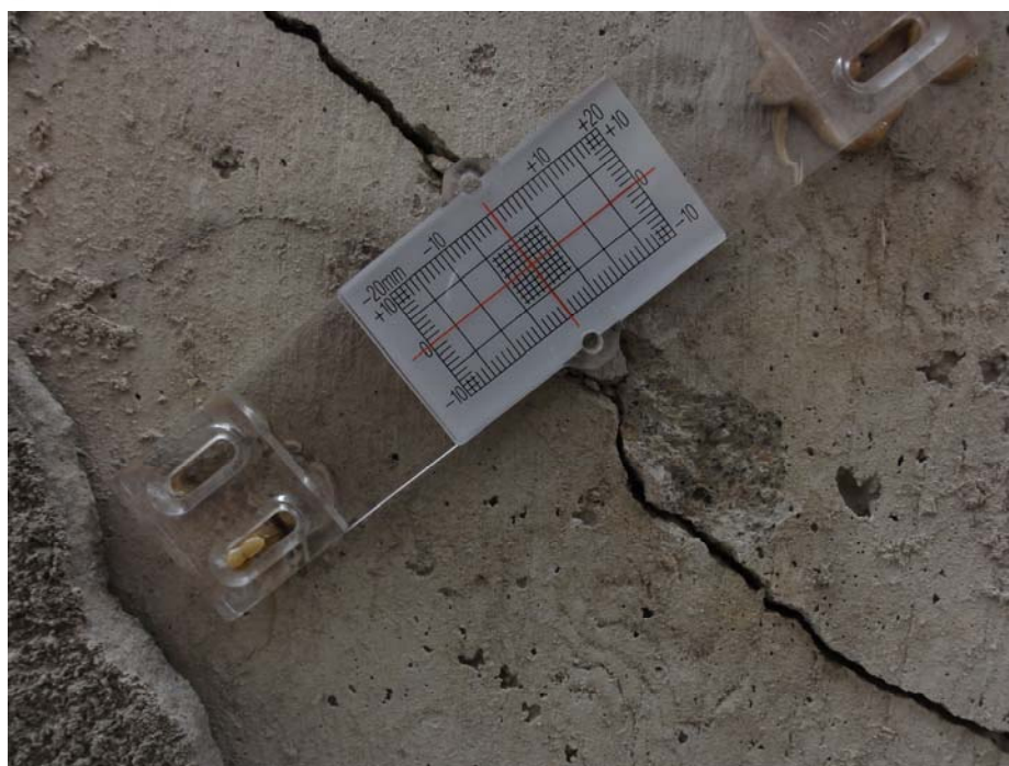
Photo F.6: Crack Meter Located on the West Face of the Retaining Wall Between 230 & 306 Sask. Cres. E. (CM3) (Sept 18, 2013)
