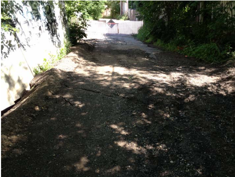
Photo C.27. Looking East at New Tension Cracking Forming on Regraded Lane (July 7, 2013)
