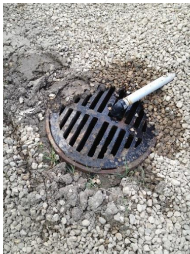
Improper storm sewer use.
