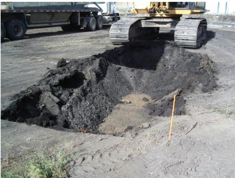
Contaminated soil at a construction site.
