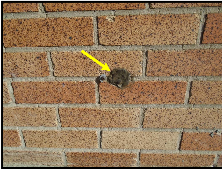
Photograph 1: Asbestos-Containing Grey Firestop Putty
