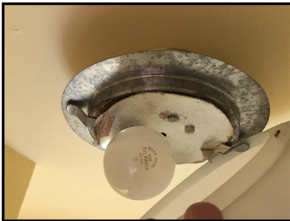
Photograph 3: Asbestos-Containing Incandescent Light Fixture Paper.
