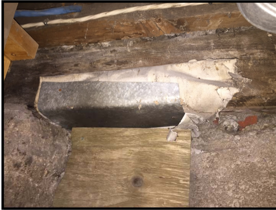
Photograph 1: Asbestos-Containing Chimney Paper Wrap.
