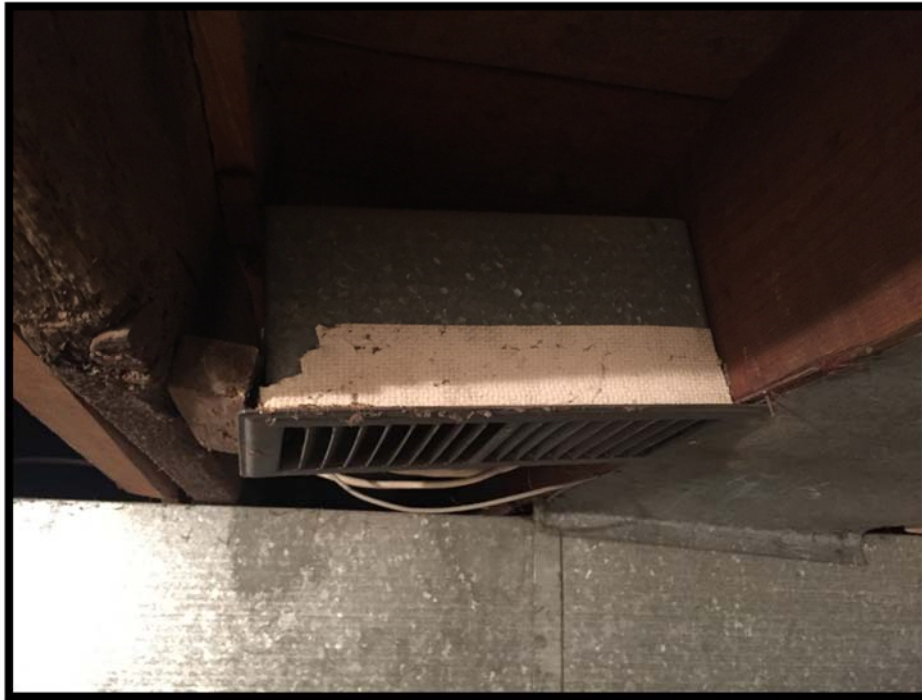
Photograph 2: Asbestos-Containing Duct Paper Wrap.
