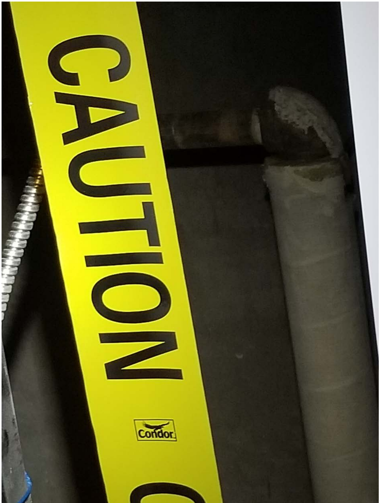
Figure 4. Elbow with Damaged Pipefitting Compound Within Ceiling Space.
