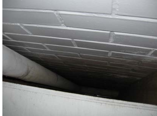
Inaccessible Pipeline Fitting
