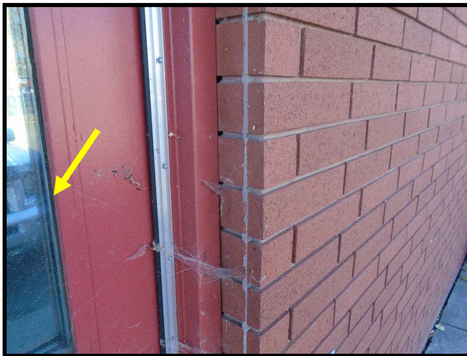
Photograph 4: Asbestos-Containing Exterior Black Window Caulking.
