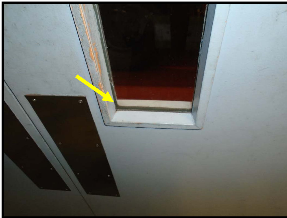
Photograph 1: Asbestos-Containing Grey Window Caulking.
