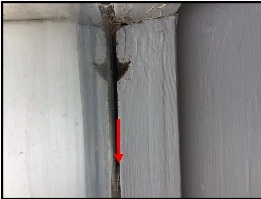
Photograph 6: Asbestos-Containing White Window Caulking.
