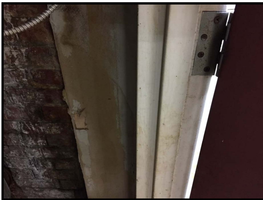
Photograph 7: Asbestos-Containing Drywall Joint Compound.
