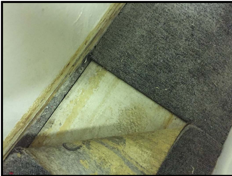
Photograph 2: Asbestos-Containing 12"x12" Floor Tile (Indistinguishable Pattern).
