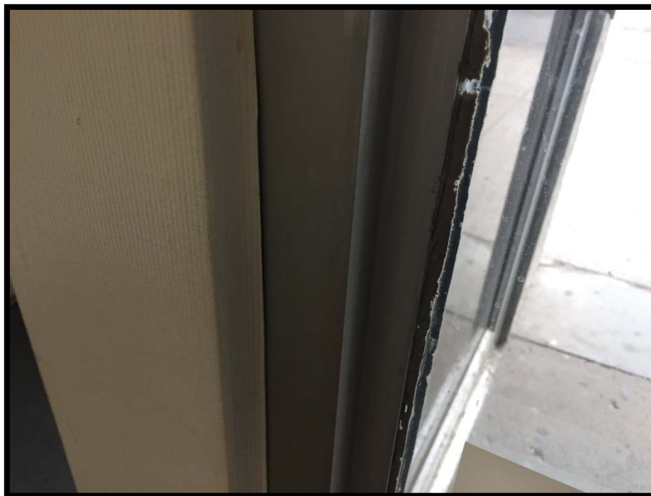
Photograph 8: Asbestos-Containing Grey Window Caulking.
