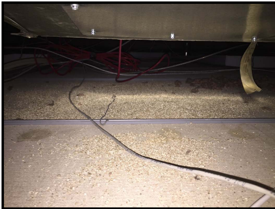
Photograph 10: Suspect Asbestos-Containing Vermiculite Insulation.
