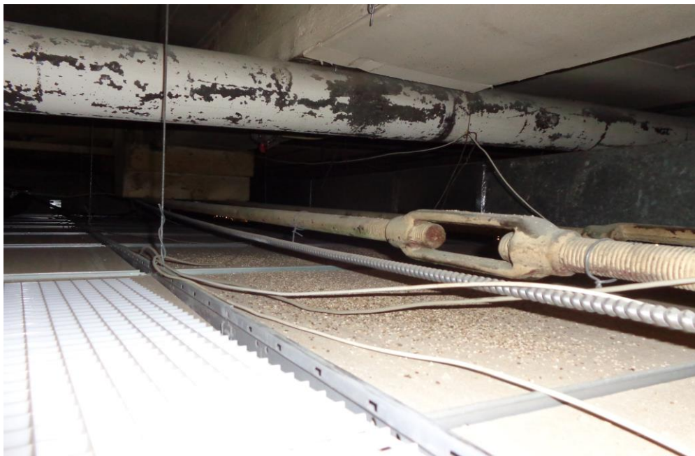
PHOTO 2 – Vermiculite Debris Within the Ceiling Space North of Meter Readers Area.
