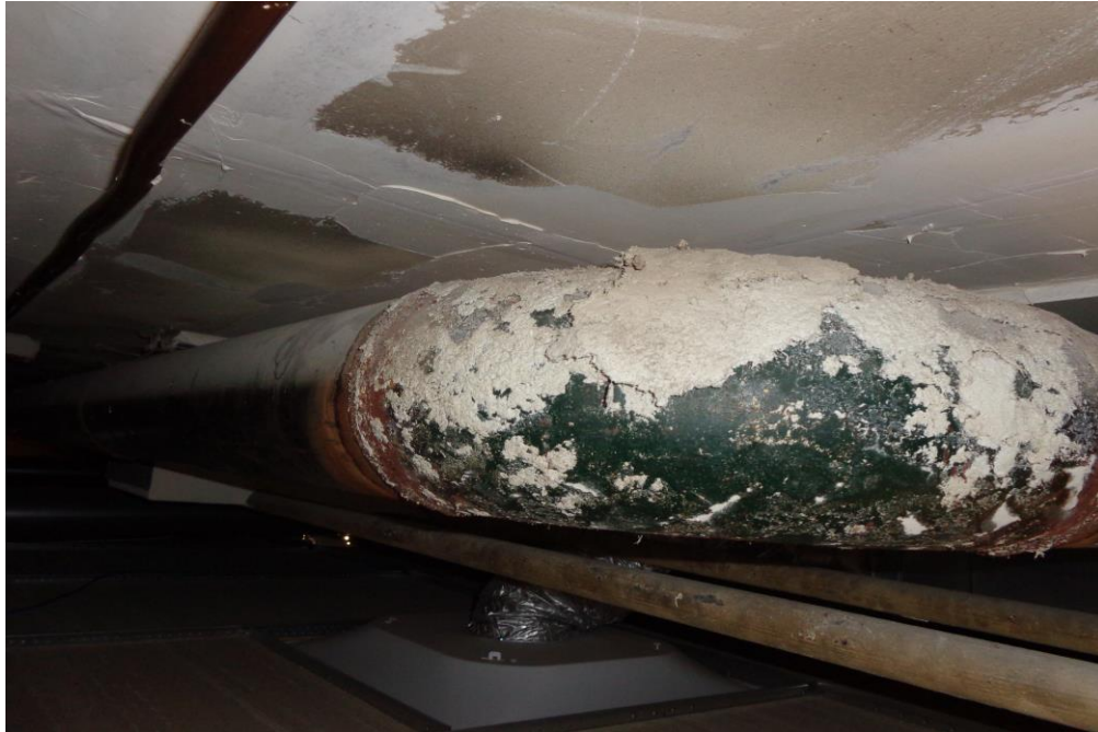
PHOTO 1 – Fire-tape on Drywall Ceiling and Remnants of Asbestos Mud Compound on Pipeline Fitting.
