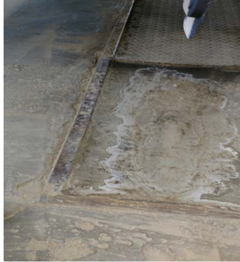
PHOTO 1 – MAIN SHOP AREA – IN-FLOOR HOIST
