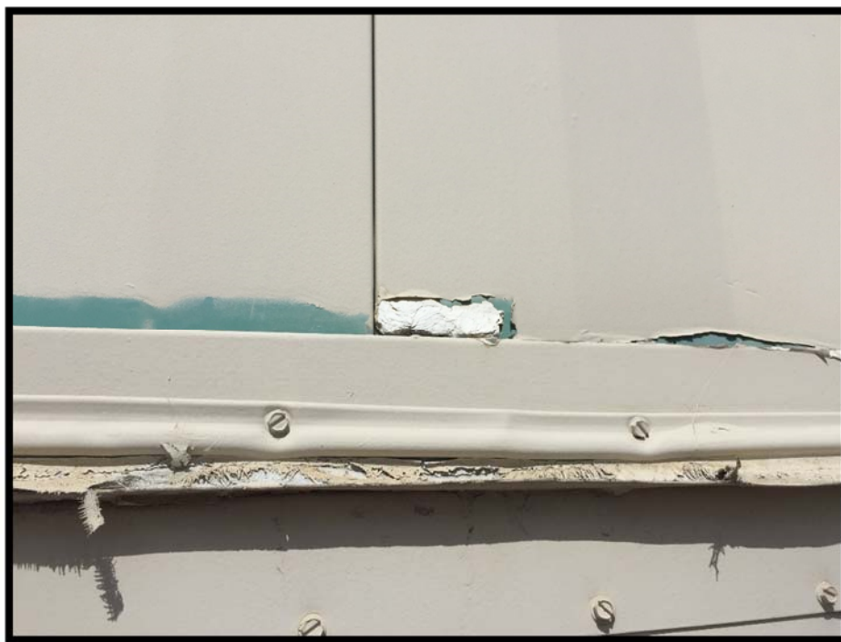
Photograph 1: Asbestos-Containing White Exterior Building Caulking.
