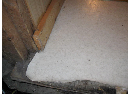
#2) Sheet Floor Covering
