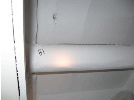
#1) Lineal Pipeline Insulation
