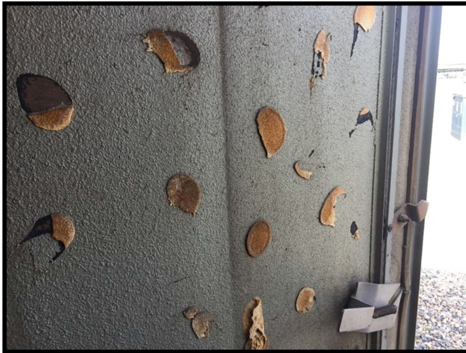
Photograph 1: Asbestos-Containing Wall and Ceiling Mastic.
