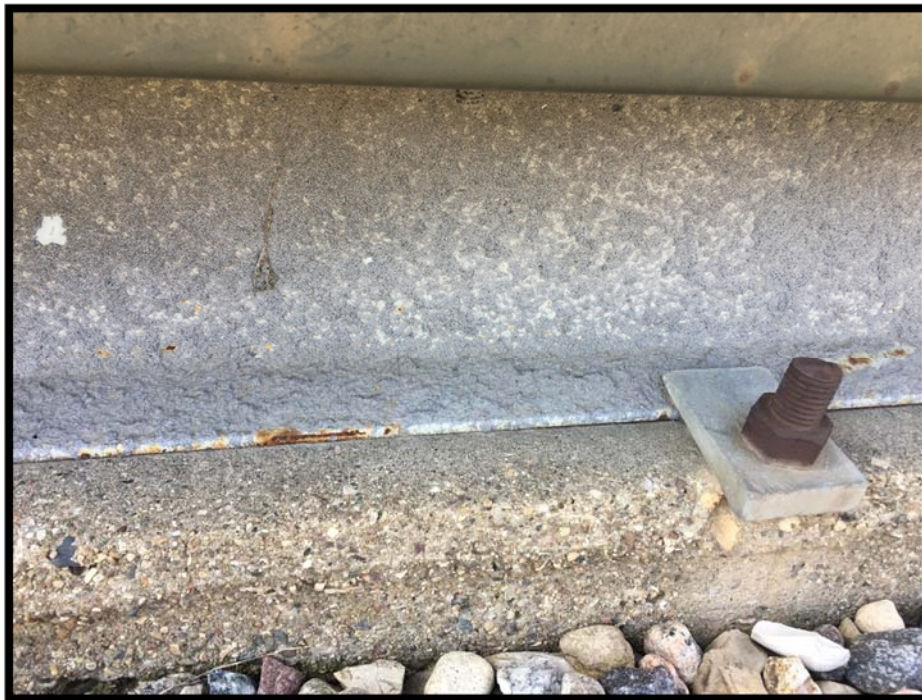
Photograph 2: Asbestos-Containing Texture Coat.
