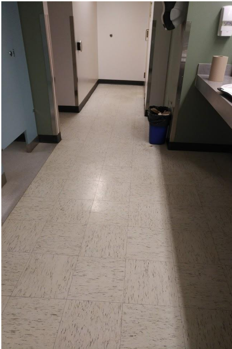
Photo 4: 209 Female Washroom – 1' X 1' Floor Tile White w Grey Streaks. Asbestos Containing Material.
