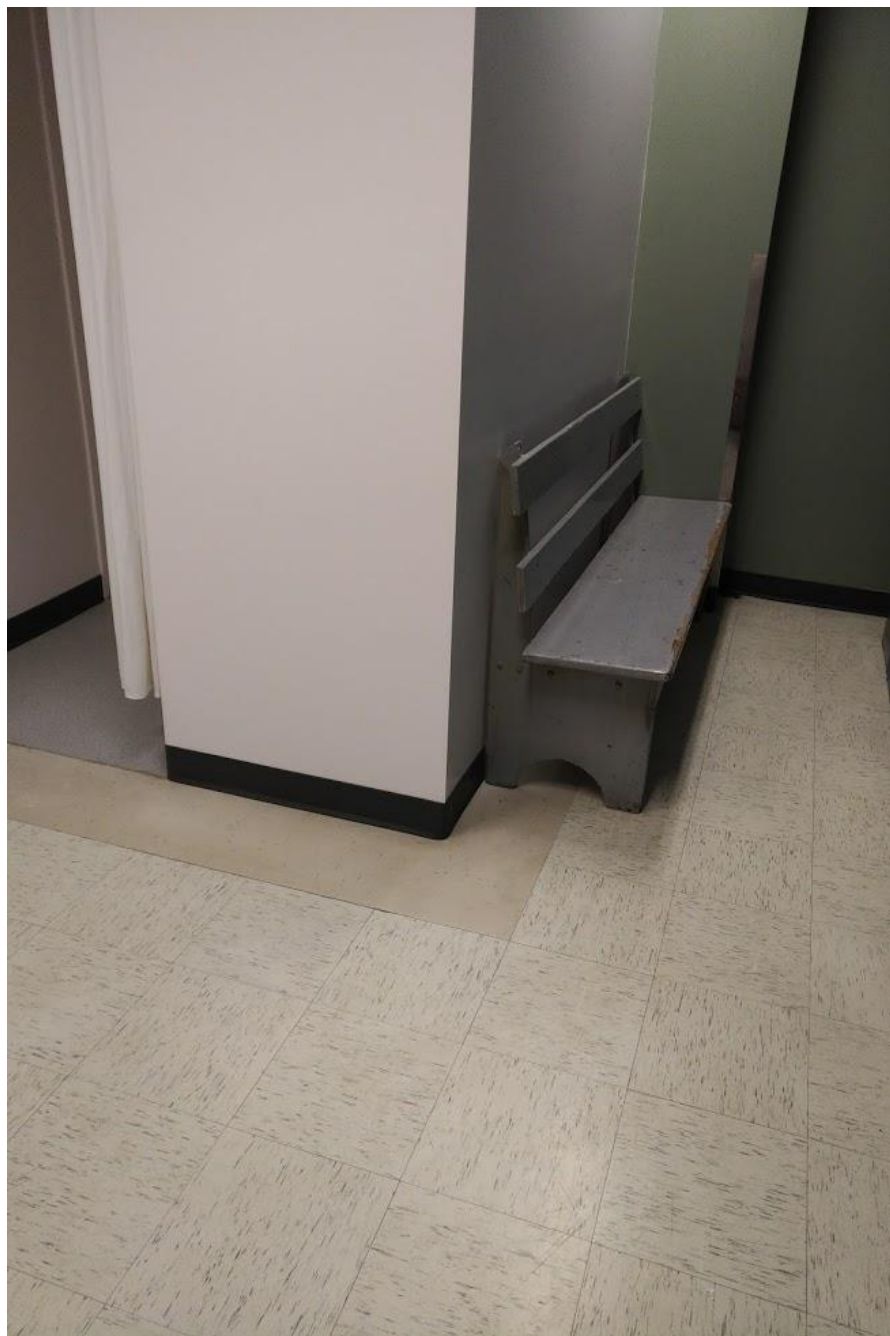
Photo 3: 210 Female Locker Room – 1' X 1' Floor Tile White w Grey Streaks. Asbestos Containing Material.
