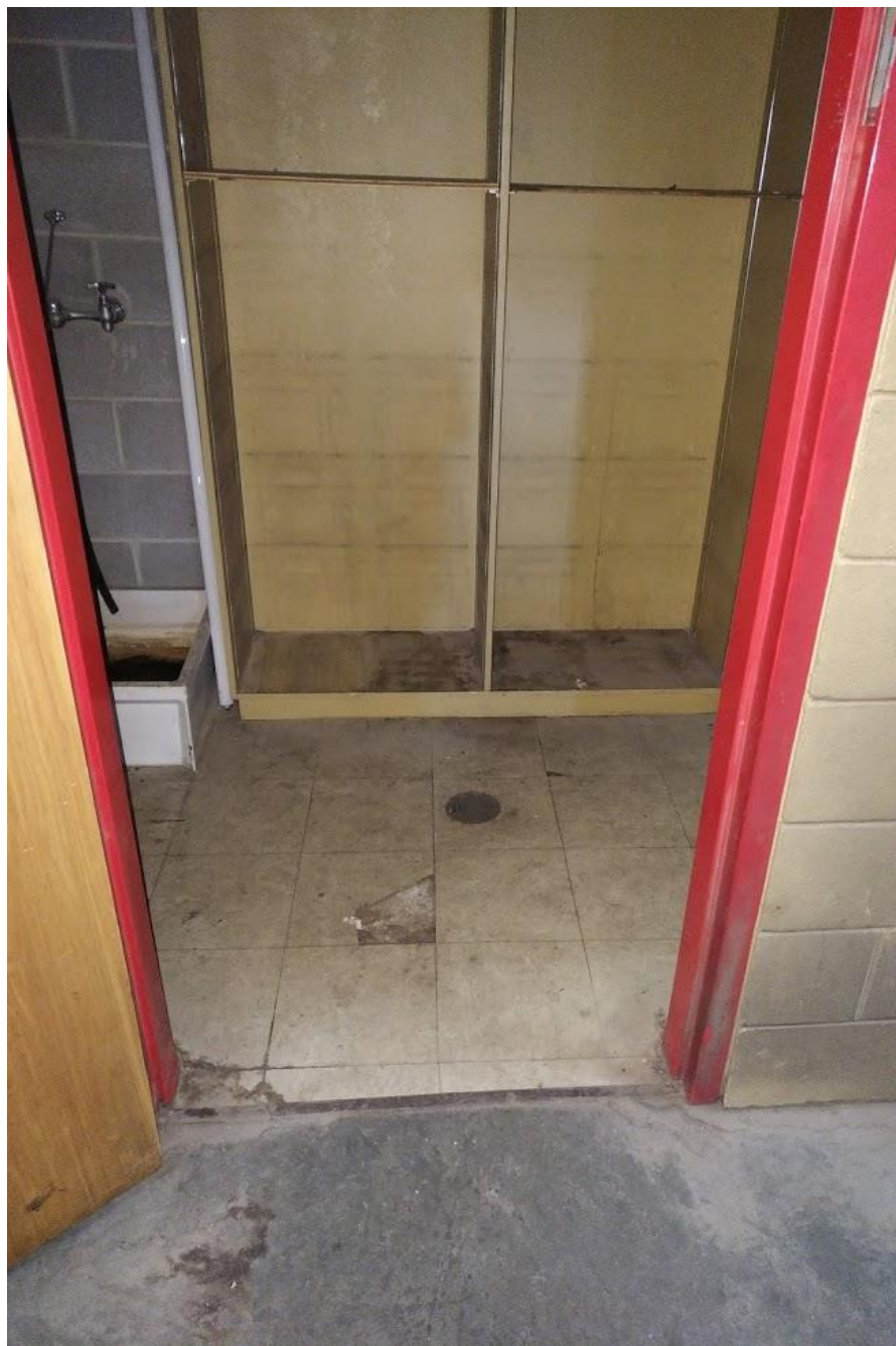
Photo 5: 122 Janitor Room – 1' X 1' Floor Tile Beige w Faint Grey Streaks. Asbestos Containing Material.
