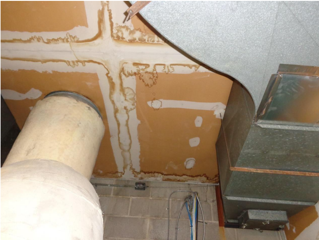
Photo 1: 225 Mechanical - Ceiling Water Staining
