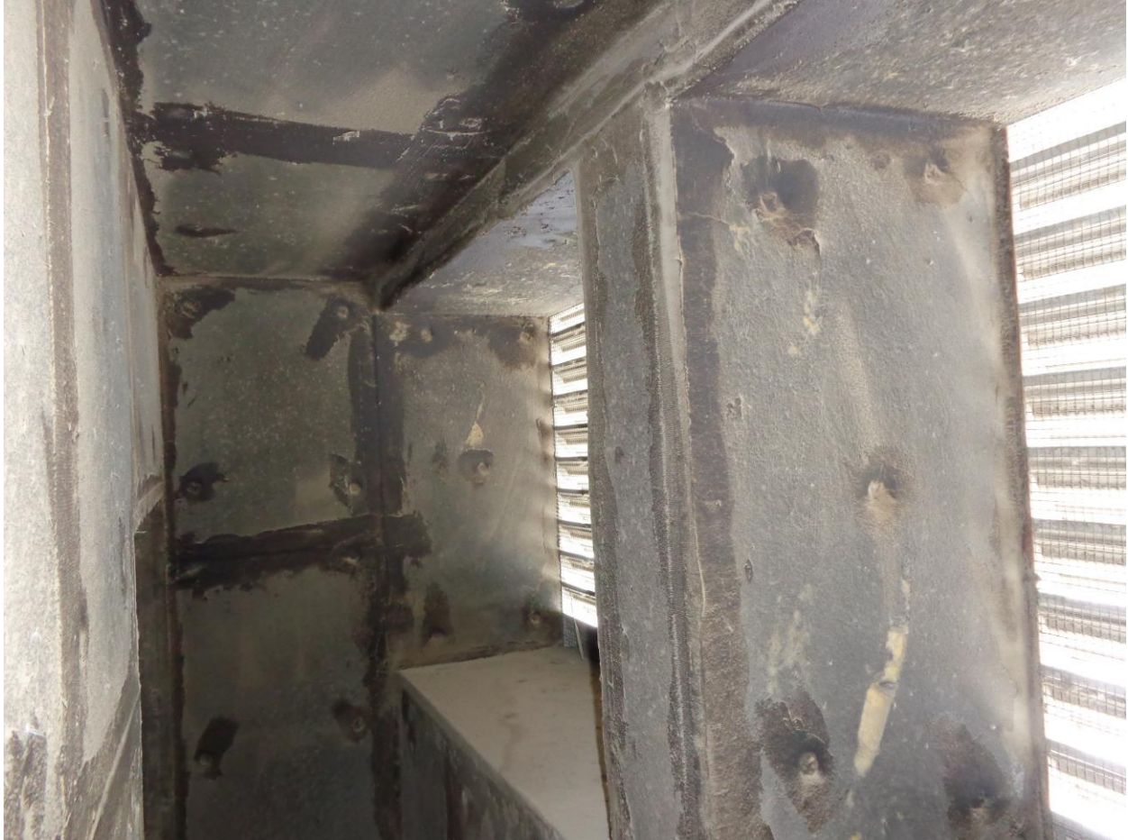
Photo 1: 225 Mechanical Room – S.A Fan S-1 Black Tar on Fiberglass Inside the Intake Air on the North Wall. Asbestos Containing Material.
