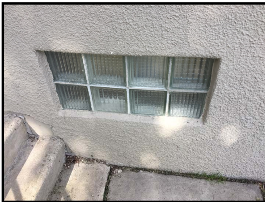
Photograph 1: Asbestos-Containing Exterior Stucco.
