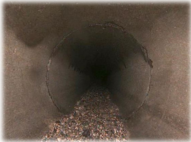
Figure 9: Image of Sediment within Storm Sewer Pipe
