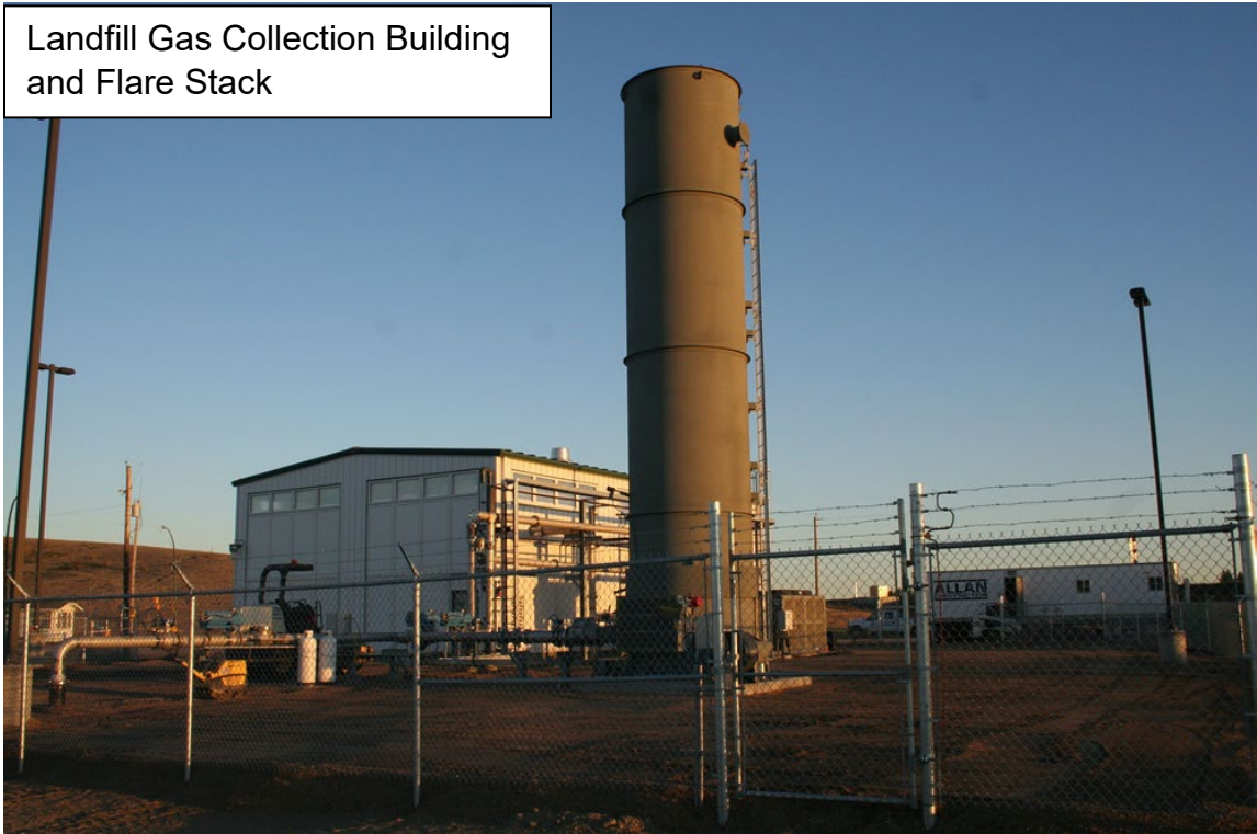
Biogas well in landfill
