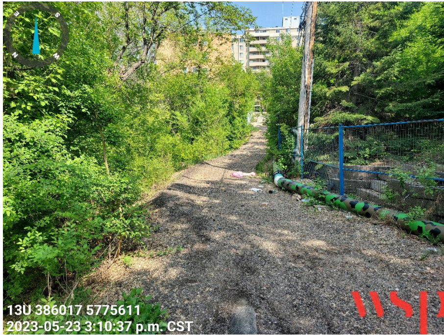
Photograph 1: Looking east down the back alley at the East Failure (May 23, 2023)
