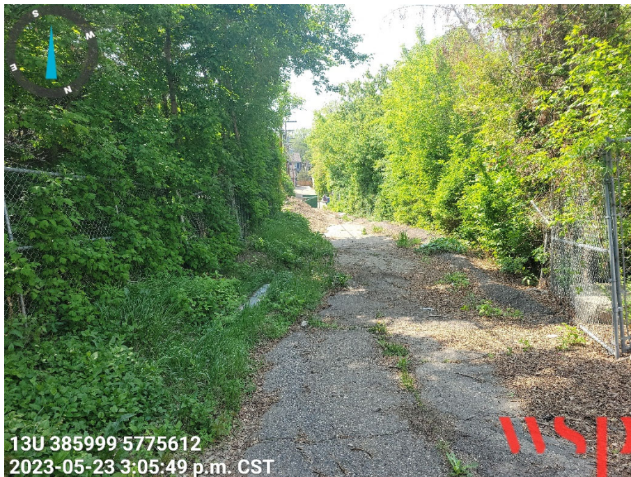
Photograph 2: Looking west down the back alley at the West Failure (May 23, 2023)
